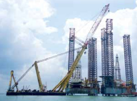
The Asian Hercules was called upon for the challenging operation to transplant the legs of Adriatic VI onto Adriatic I which was completed on time, safely and on budget
